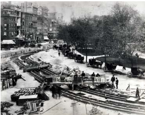
Construction of the railway next to Madison Square Park after 1890 (From the Baruch College Archives)
